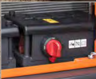
Battery cut-off switch
